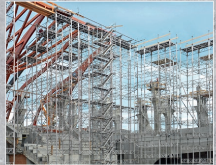
Access & Safety platforms
